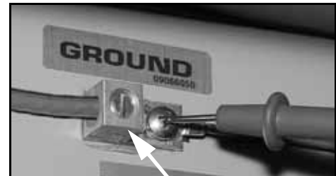
Water Heater Ground Connection
